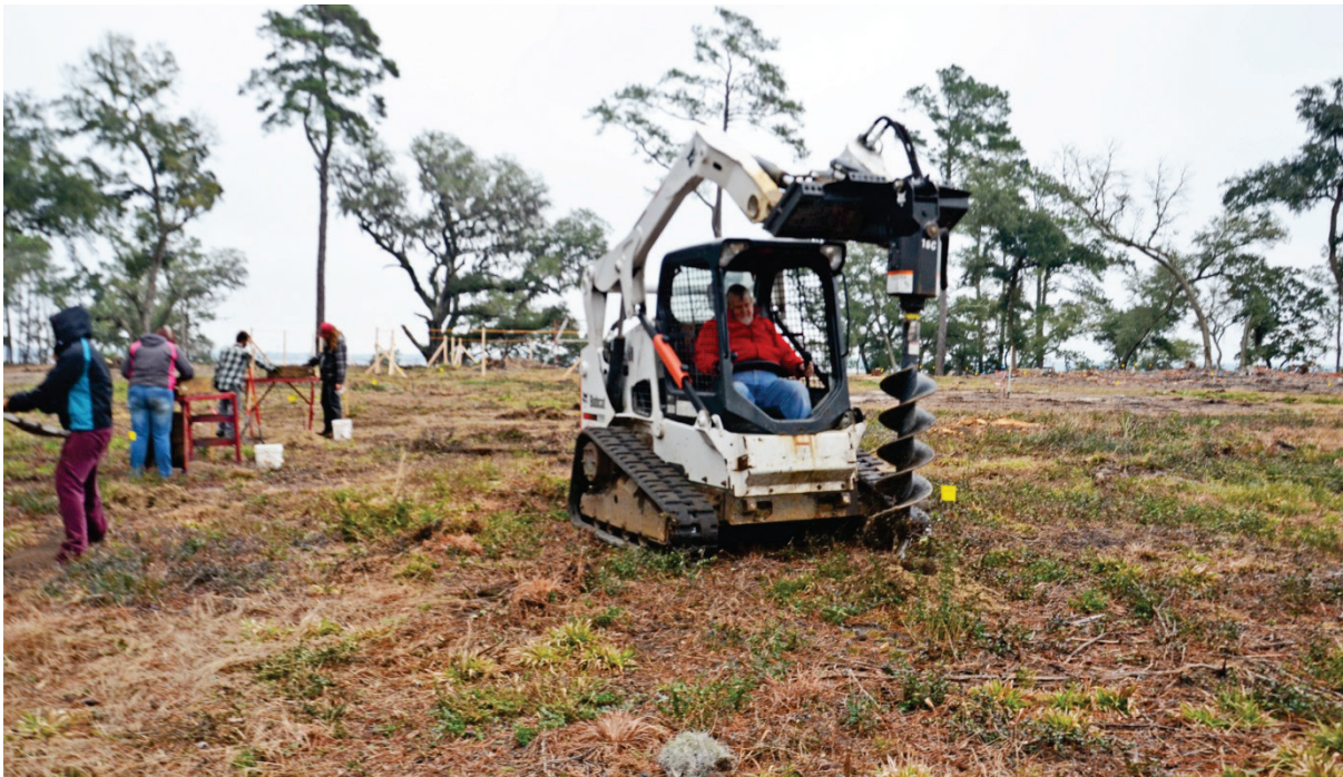
Figure 30. Site clearing and auger testing. The upper photo shows the Kendal site cleared of vegetation and initial efforts to remove loose brick to reveal structural details. The lower photo shows auger testing and screening of the tests.
