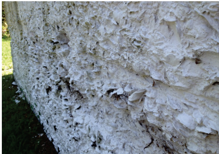
Figure 82. Upper photo shows shell inclusions in mortar. Lower photo shows a tabby wall built in lifts or pours (upper photo courtesy of Sidney Living Museums, New South Wales; lower photo courtesy of Wikipedia).
