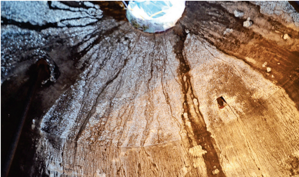
Figure 59. Feature 4, cistern. Upper photo shows the sandstone cover recovered from the bottom of the cistern. Lower photo shows the domed roof of the cistern. On the right is the entrance from Feature 1, the initial feature. On the left is a pipe whose function is uncertain.
